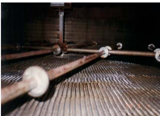
Vacuum GasOil Draw After Decontamination
